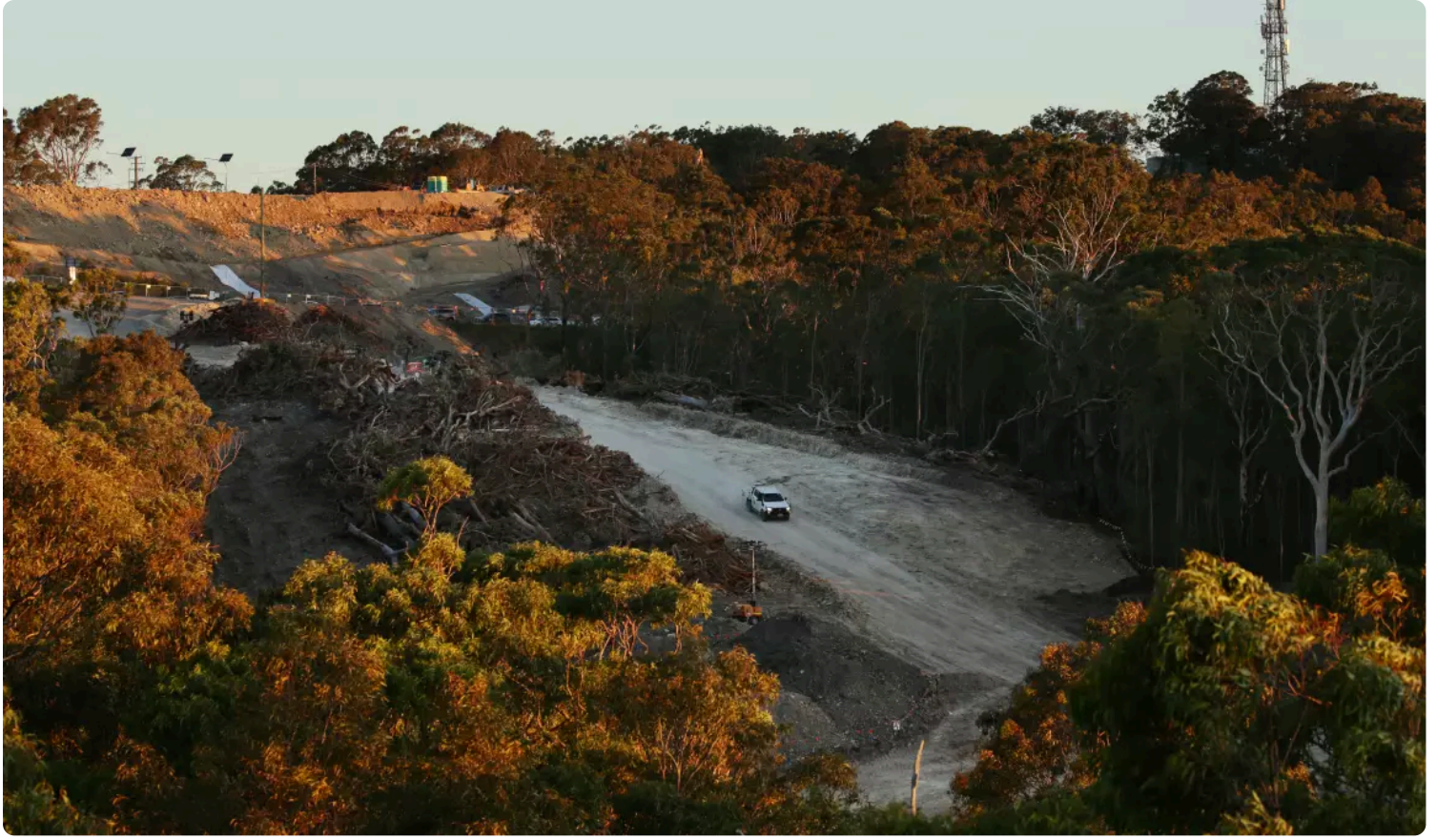
📷 Early construction of the Newcastle Inner City Bypass in mid-2023. Picture by Simone DePeak.
